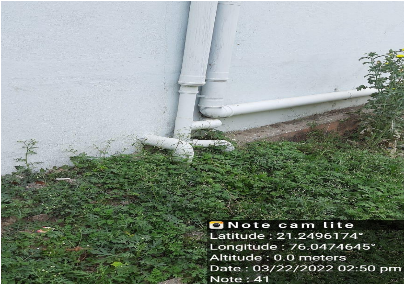
Water Purifications Waste Water Harvesting
